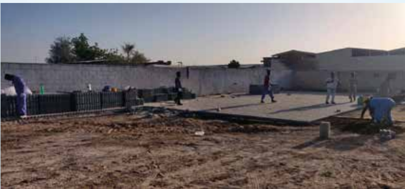
Construction of Office, Accommodation Room, Ablution Area, Interlock Flooring & Steel Structured Warehouse at Al Ain for M/s. Madar Emirates For Building.
